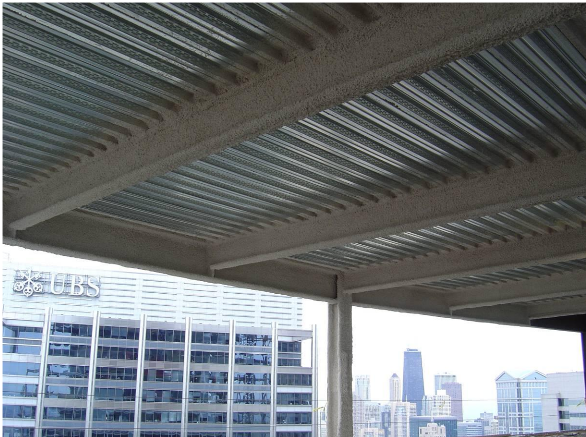
Sprayed fire protection
